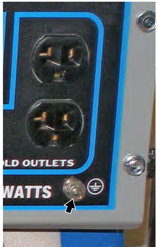
Figure 12 – Ground Terminal on the Control Panel
